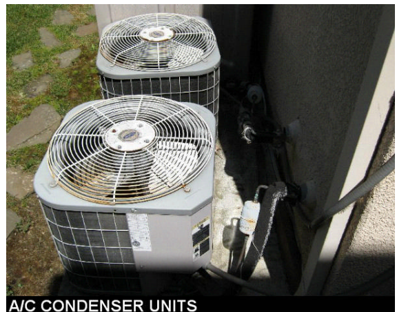
A/C CONDENSER UNITS
